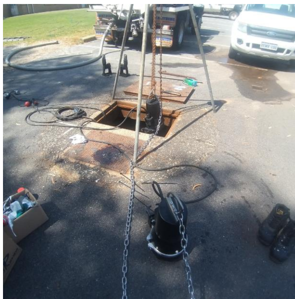
Pump installation and new chains
