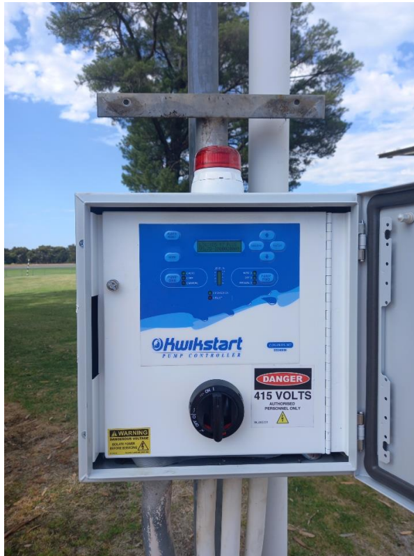
New Control Panel
