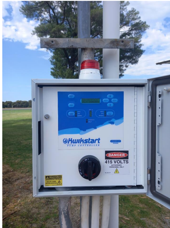
New Control Panel
